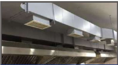
Exhaust And Fresh Air Duct
