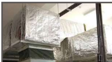
Acoustic Insulation Service
