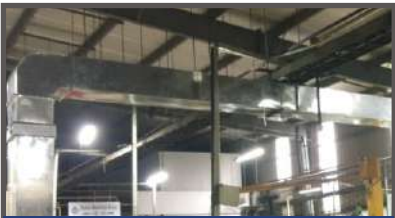
Fume Exhaust Ducting
