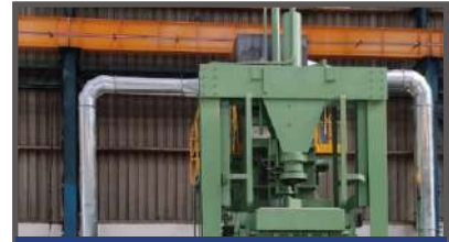
Round Duct Work
