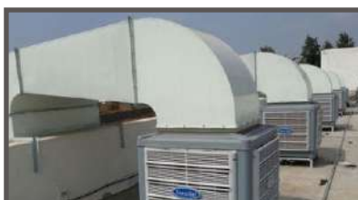
Air Cooler With Ducting
