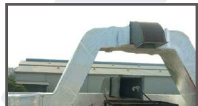
HVAC Ducting Insulation Service
