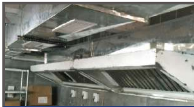
Fresh Air And Exhaust Ducting System
