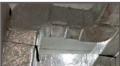
Duct Thermal Insulation
