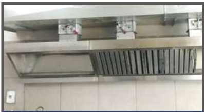
Kitchen Exhaust System
