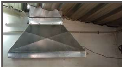
Kitchen Exhaust System
